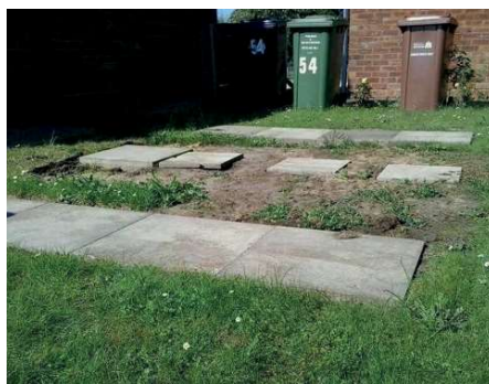
Not level due to sub soil movement beneath ground and gaps between the slabs.
