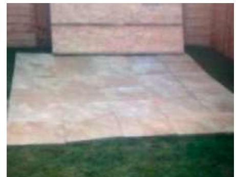
Unevenly lying slabs directly on top of a lawn.
