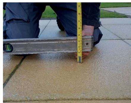
An unlevel base means the structure walls will not sit square to the floor. This will cause the structure to be unsecure and pull apart over time.
