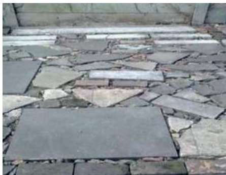
A mixture of broken slabs with no cement filled gaps.
